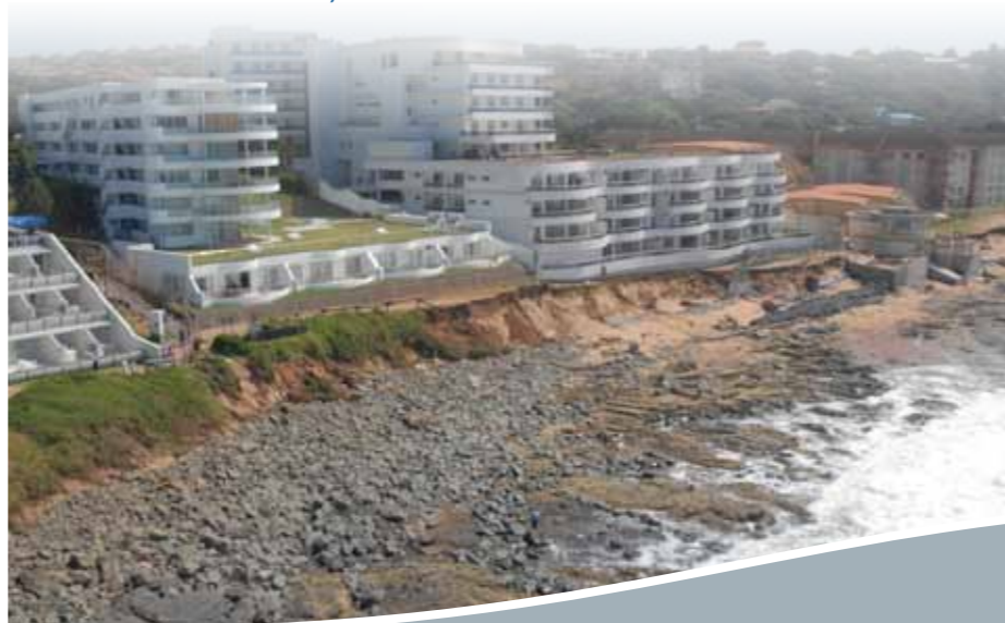
Erosion at Willards Beach, Ballito in KwaZulu-Natal after March 2007 storms
